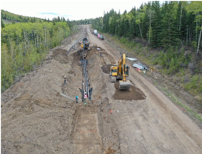
Sewage Treatment Plant Road closed for construction of the new Wastewater Treatment Plant.
