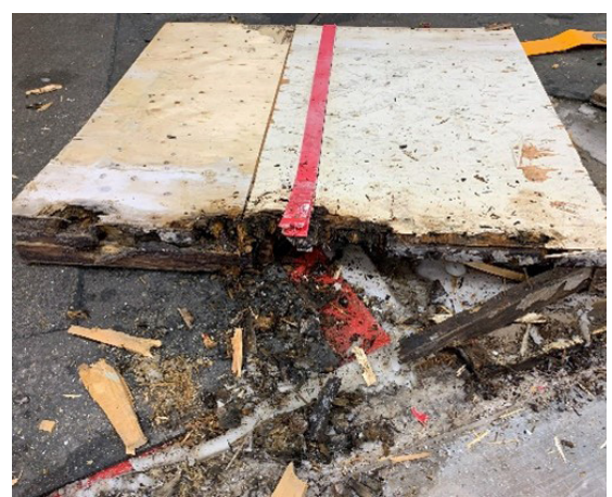
Photo shows poor condition of the former boards.
