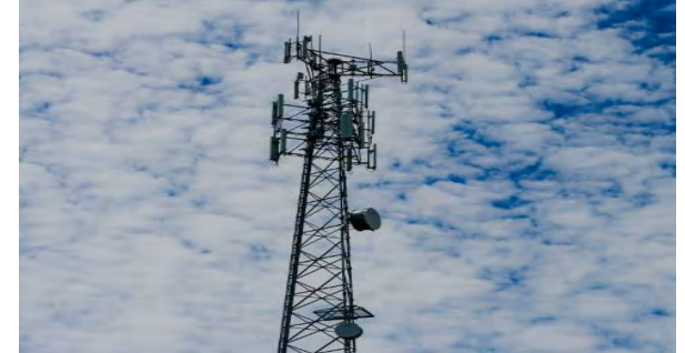
Telecom & Cable Distribution
