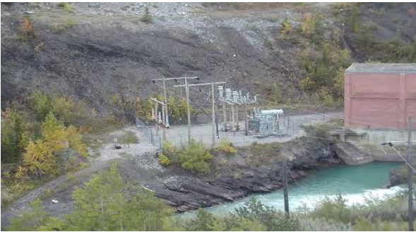
Electric Power Systems
