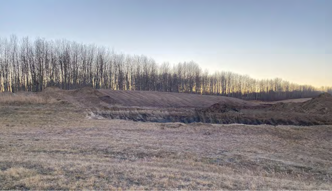
Photo Description: Water Pit developed on East Boundary of lot South of the Traffic Bulb. Facing Southwest. Requiring update to the Storm Water Management Plan:
